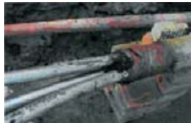
Fig. 2: Corrosion on the outer sheath and the building of holes in the lead sheath
