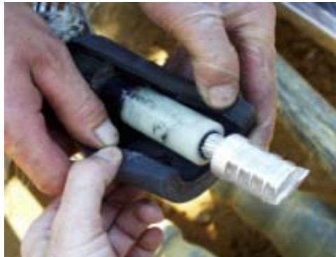
Figure 1: PD surface traces on the improperly removed insulation shielding
