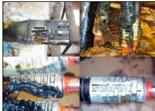
Figure C1: Fault cause analysis of disturbed cable termination. Several sharp edges on the connector were found on all three phases.
